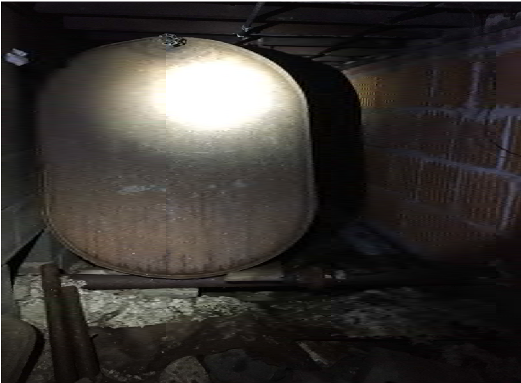
Above ground heating oil tank - 275 gallon in basement of school building
