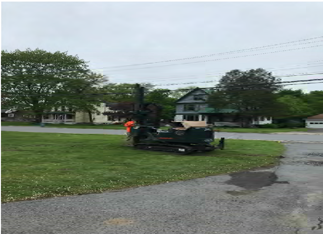
Installation of Soil boring SB-6 at northwest corner of the site (looking west)
