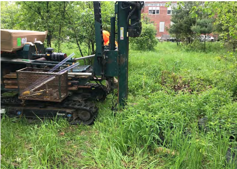
Installation of Soil boring SB-8 / monitoring well MW-2 in rear yard area
