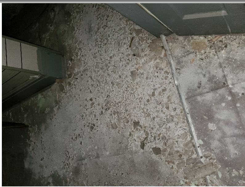
Material 23020-001 9" x 9" Floor Tile This material is present beneath non-ACM plaster debris and guano.
