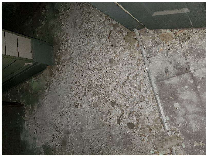
Material 23020-001 9" x 9" Floor Tile This material is present beneath non-ACM plaster debris and guano.
