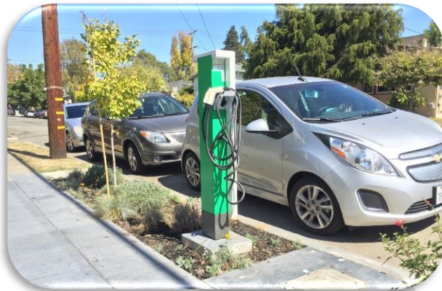
Curbside Charging; Image Source: https://www.berkeleyside.org/2016/09/22/curbside-electric-vehicle-charging-stations-start-to-appear-in-berkeley
