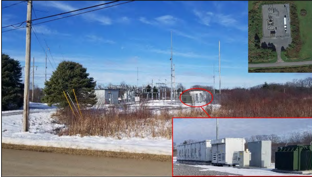
The Pulaski small, 2 MW battery energy storage system, designed to sustain a 2,000-kW customer demand, as seen from the road. The top right portion of the image shows an aerial view of the storage system (source: Google Earth Pro). The bottom right portion of the image shows the storage system up close (source: NYS Tug Hill Commission).
