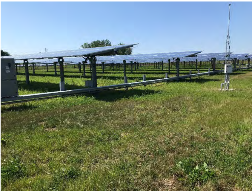
Solar installation in Seneca County which shows the above ground infrastructure, which could present problems for mowing or sheep grazing. Photo: Joe Lawrence
