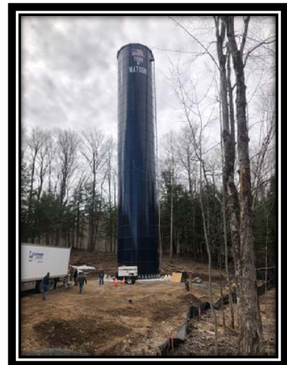
Picture: Town of Watson Drinking Water Storage Tank Water District #4 Ext. #1
