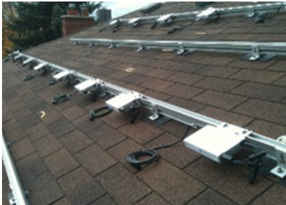
A Solar Electric Racking System
