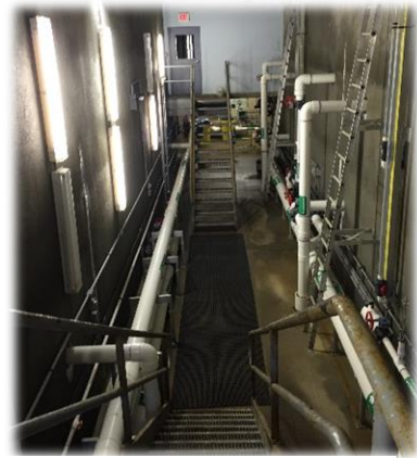
Picture: Water Plant Pipe Gallery
