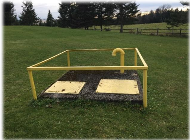
Picture: Well pit
