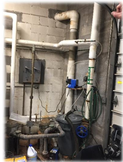
Picture: Chlorination inside building
