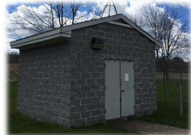
Picture: McAlpine Street pump station
