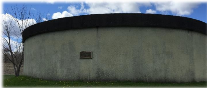
Picture: McAlpine Street 200,000 gallon storage tank
