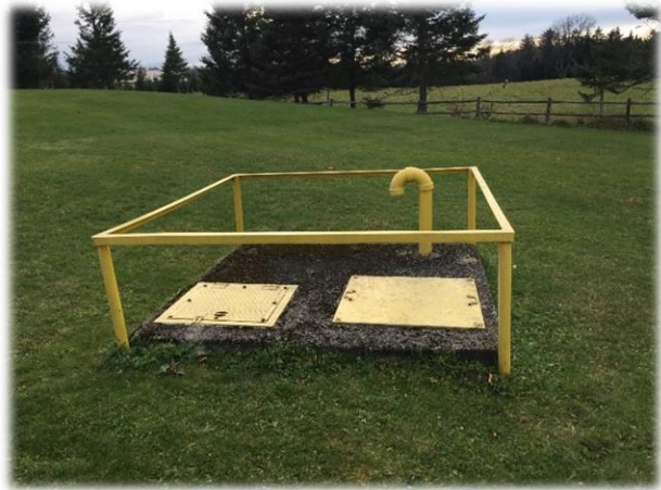
Picture: Well pit
