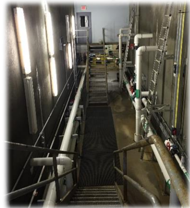
Picture: Water Plant Pipe Gallery
