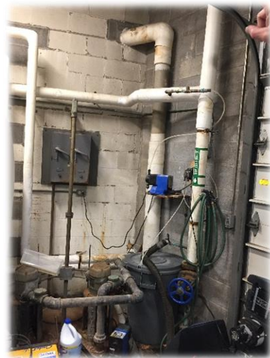
Picture: Chlorination inside building
